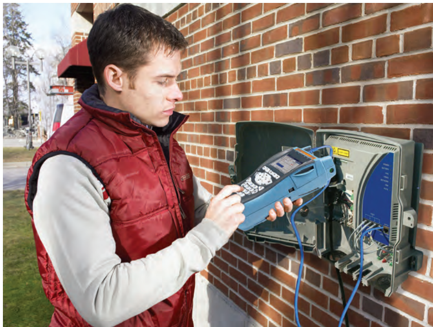
Testing IPTV at the Ethernet port of the ONT.
