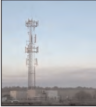
Typical Cell Site
